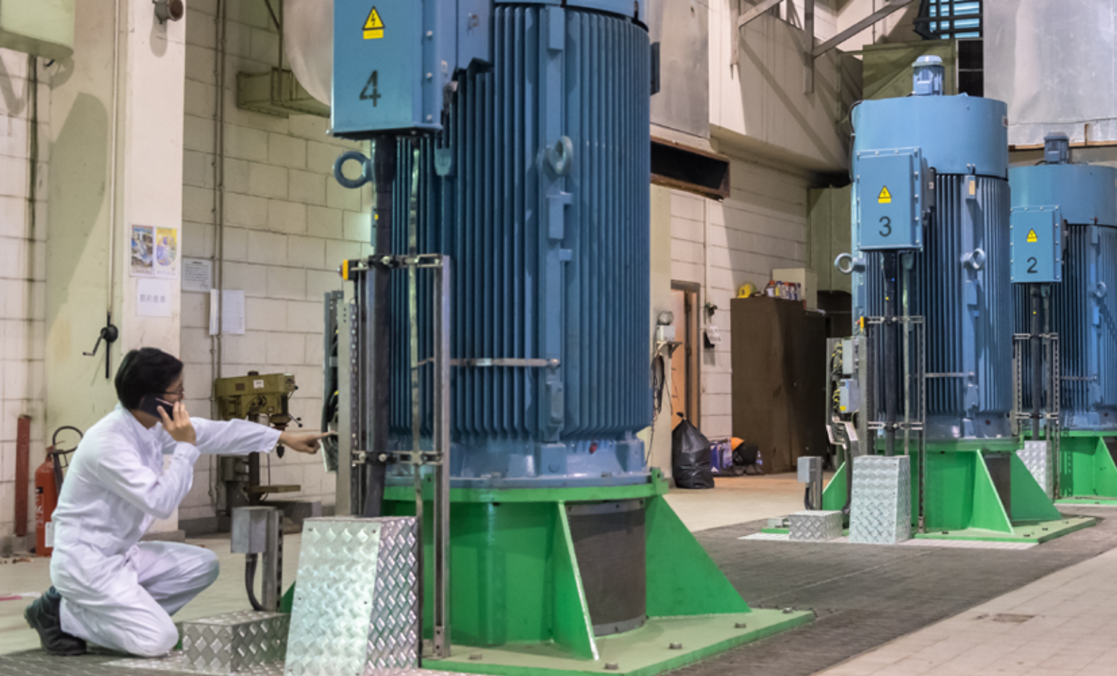
Sha Tin Sewage Treatment Project in Hong Kong, China. Photo: Asian Development Bank
